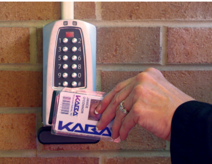
Stand-alone access controller located at front entrance.
